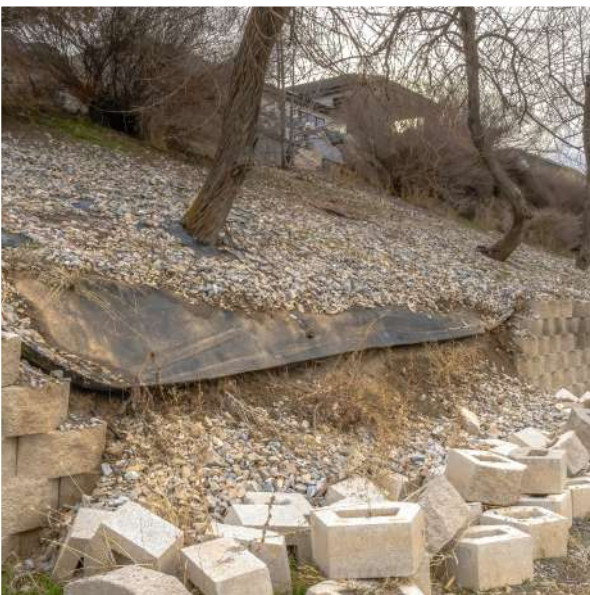
WITH NO GEOGRID INSTALLED
